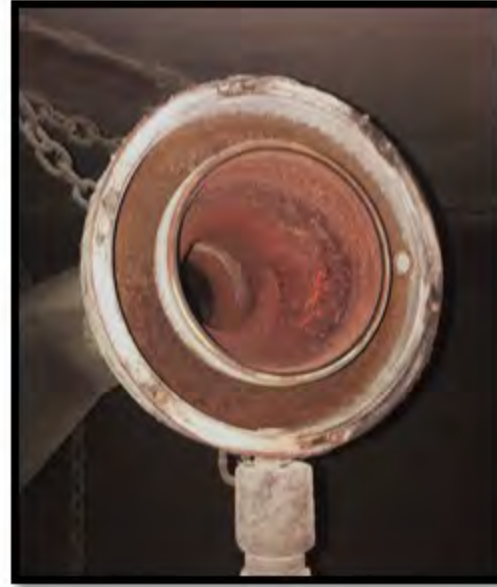
There is a high level of surface rust on the sound generators. However, the wear surfaces are within tolerance.
