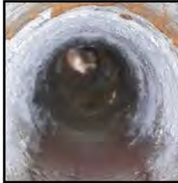
Close up view of the ID of the acoustic cleaner's bell sections.
